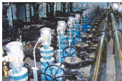
The SUPER SHREDDER in an arsenal configuration protects a major metropolitan wastewater facility.
